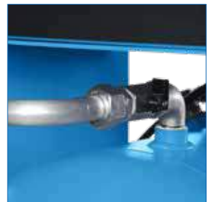
Flexibility to bypass dryer
