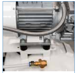
Pump unit mounted on anti-vibration devices
